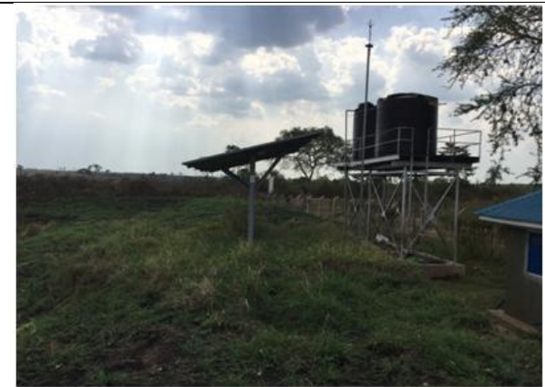
b) Solar powered water pump at the site- Gangama village
